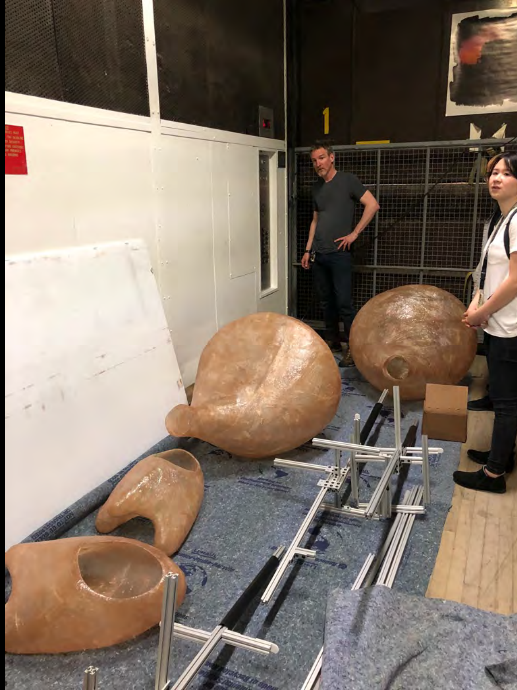
Beginning assembly TJ McLeish, Master Fabricator Wendy Wu, MFA IxD Class of 2019
